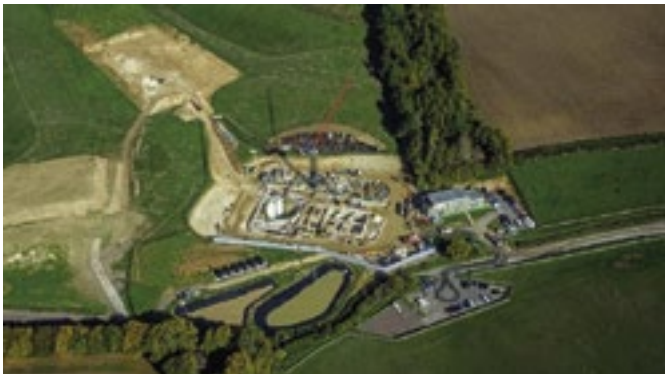
The Chalfont St Giles vent shaft at the top of Bottom House Farm Lane
