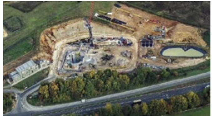
The Little Missenden vent shaft alongside the A413
